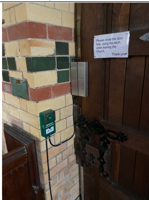
Door closed, configuration of electromagnetic mortice lock, opener and break glass override
