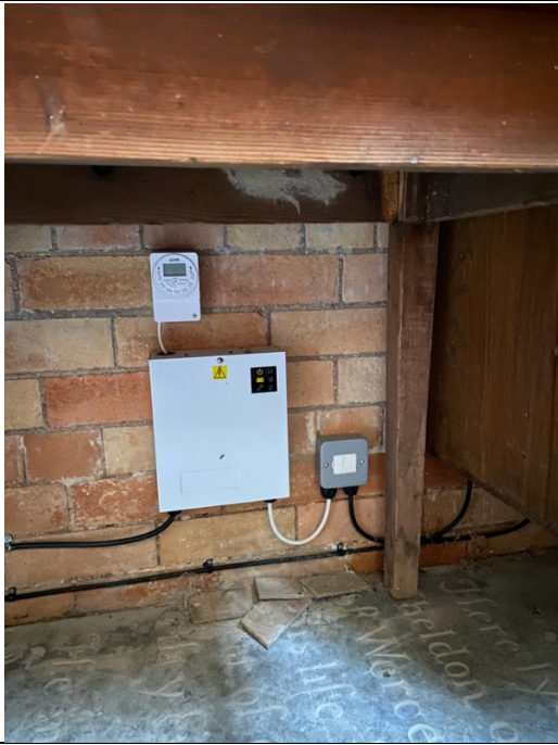
At the rear of the church, to the left of the Mains Consumer Unit, step down transformer and timer for the electronic lock
