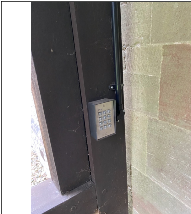
Key pad – on the outside of the main door and to the left
