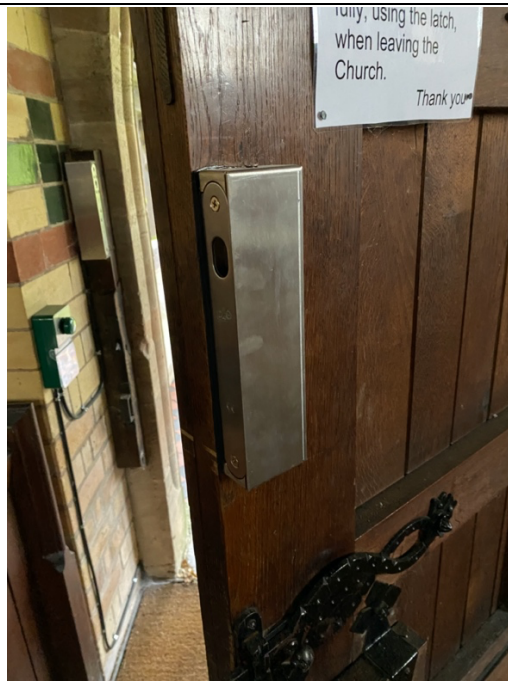
Inside the main door, open. Electronic mortice lock fitted to the frame, the receiver on the door.
