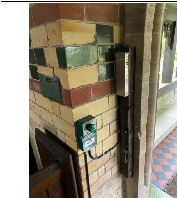
Door open, configuration of electromagnetic mortice lock, opener and break glass override
